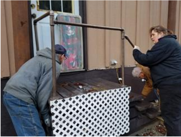
John Boy Delaney, Verne Blalack and Krista Kirby reset the stairs under the back door after the trailer skirting is installed there.
