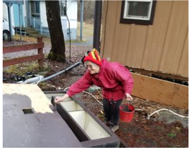
Judy Blalack stains the skirting panel before it is placed behind the front steps.
