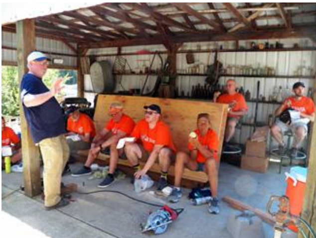
Jim Taylor of Taylor Made Construction teaches the cyclists how to construct the deck flooring for the Riley home.
