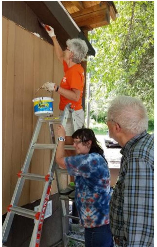
Verne & Judy brought one of Pastor Nick's ladders from the Curtis site to finish the close work on Krista Kirby's trailer home where Ginny Hughes, from Massachusetts, stained the eaves. Sonya Siedschlag from the Grace Evangelical Free Church spent hours steadying ladders for her. Ginny hoped to see Krista since she worked on this home last year, but sadly Krista had to work.
