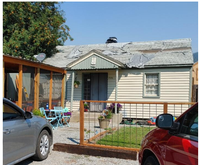
Here is our first view of Luke & Caroline Prince's roof in August after the January windstorm. The tarp had rotted away.
