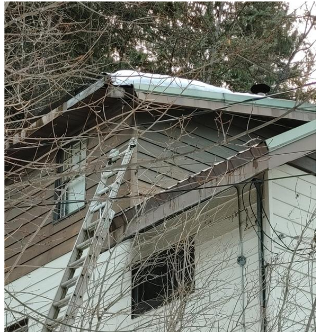
This photo is of the broken corner of Donna Marquette's roof last March. It had been damaged for two years.
